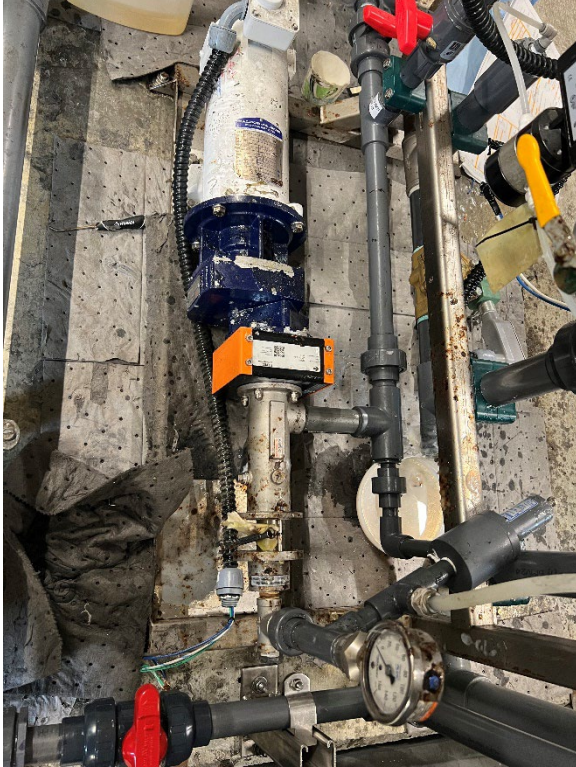
Original Chemical Metering Pumps
