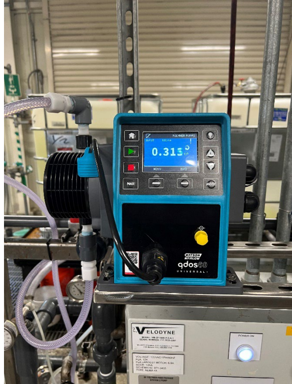
New Chemical Metering Pump
